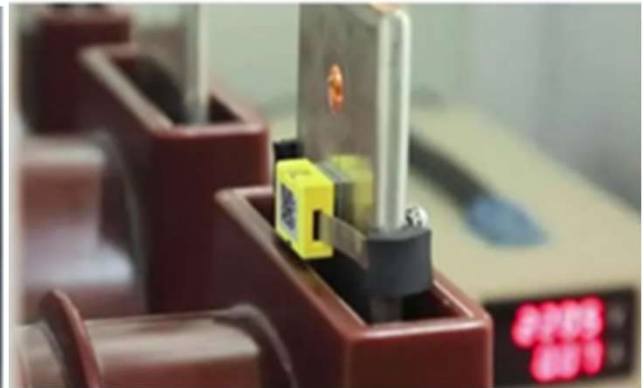
Installed on Busbar of switchgear
