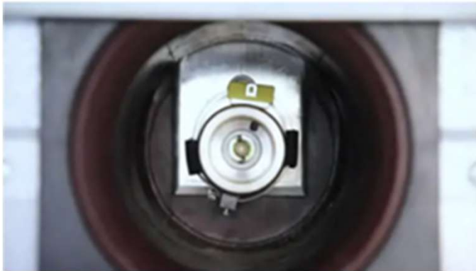
Installed on Fixed Contact of switchgear
