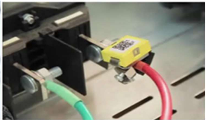
Installed on Cable Joint Drawer
